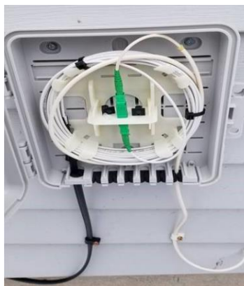
Figure 2 Baseline TAP Box Installation
