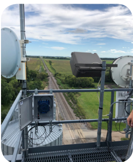
Clearfield's YOURx Flex Box with Clearview Blue Cassette, FieldShield FLATdrop and fiber jumpers installed on top of a grain elevator.
