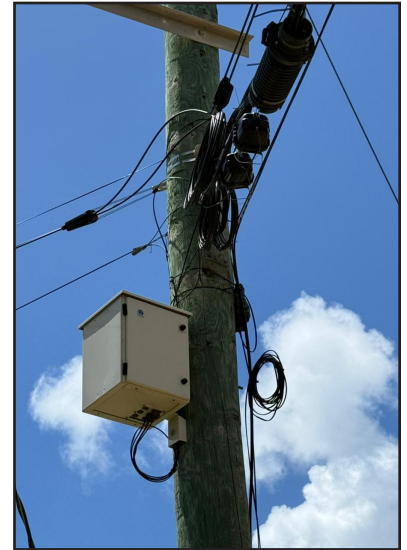
Clearfield FieldSmart® Fiber Distribution Hub (FDH) cabinets equipped with Clearview® Blue Cassettes support CCT's network needs.
